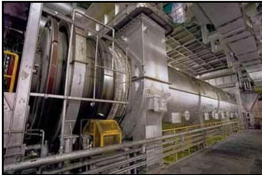
Figure 4.4: Photo of the EDDITH Rotary Kiln at Izumo, Japan
