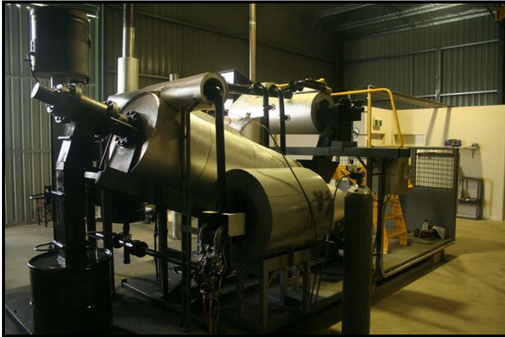
Figure 4.13: Picture of 200kg/h BES Pyrolysis System
