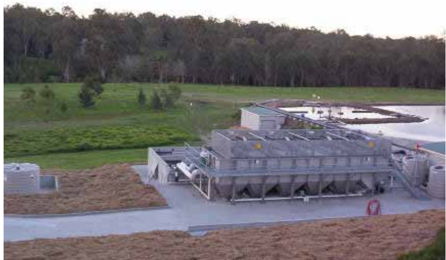
Tertiary treatment of effluent using dissolved air flotation cell
