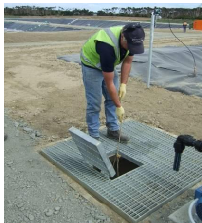
Photo 10: CAL outlet sampling point
