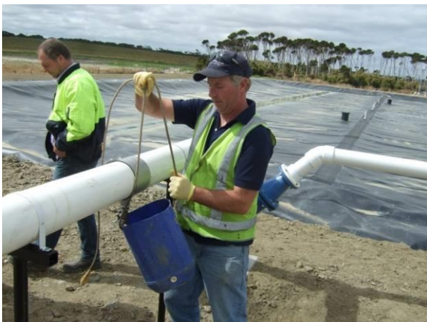
Photo 9: CAL inlet sampling point
