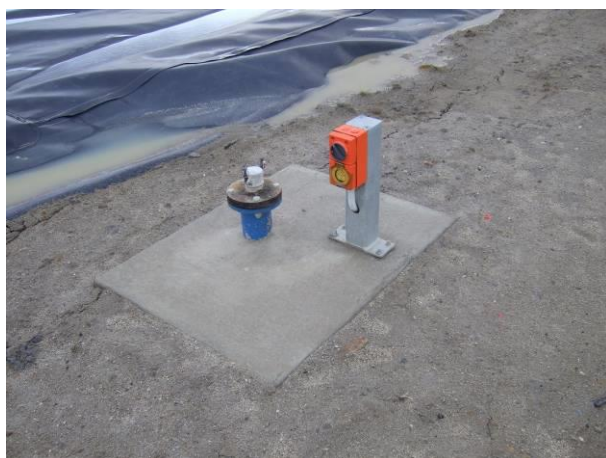
Photo 6: Sludge pipework upstand
