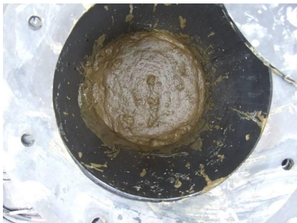
Photo 17: CAL crust at flare end
