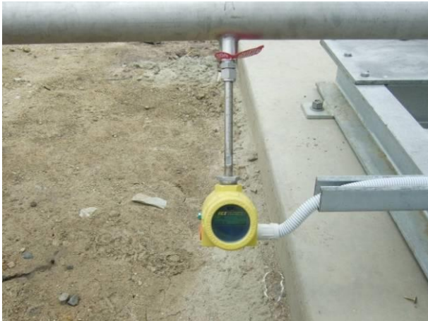
Photo 11: Inline FCI biogas flow meter
