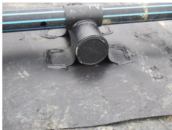
Photo 7: Sludge pipework weights
