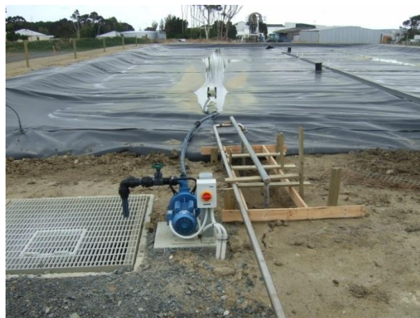
Image 12: Typical stormwater removal system.
