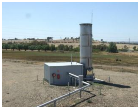
Image 6: Fully enclosed flare treating CAL biogas
