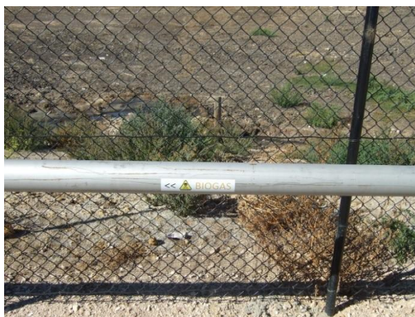
Image 13: Above ground stainless steel biogas pipe
