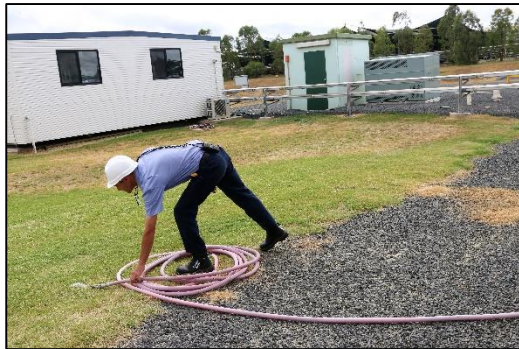
Inground knockout pot to collect condensate Image: NB Foods, Oakey
