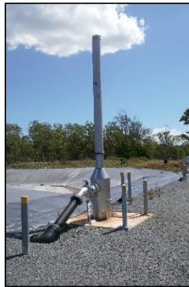
Water seals or hydrostatic valves Image: Teys, Beenleigh
