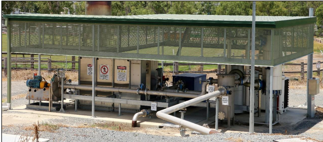
Pipeline from CAL delivering biogas: Stainless steel knockout pot(right) to blower (left)
