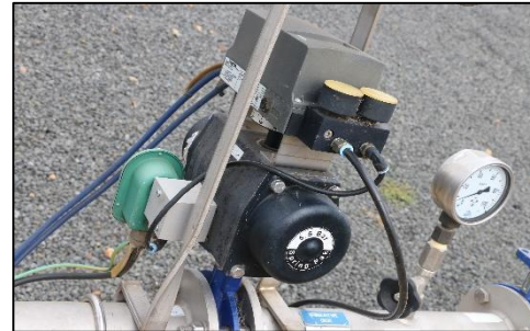
Shut off system Image: NB Foods, Oakey
