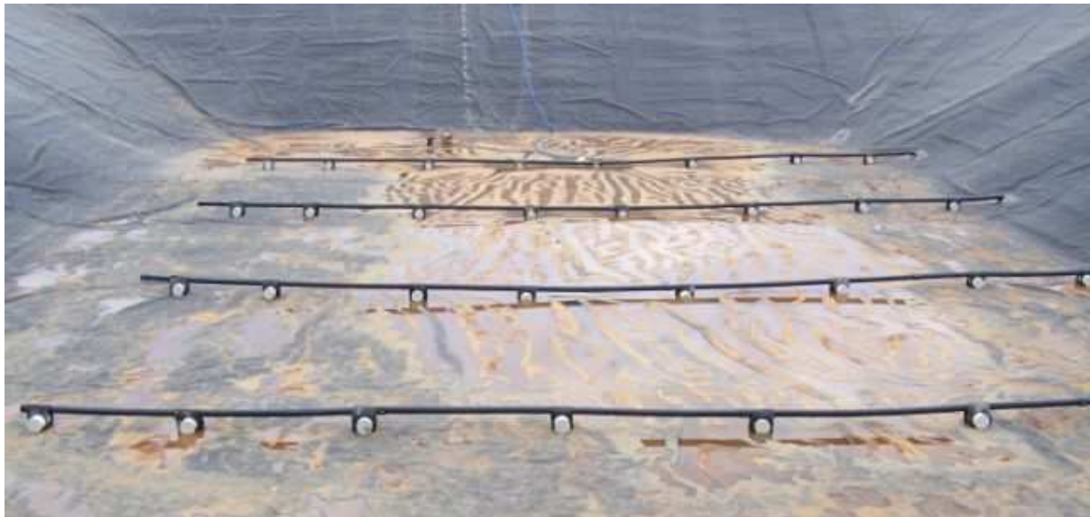
Figure 5: Sludge Removal Pipes, A J Bush Riverstone (Source: A J Bush)
