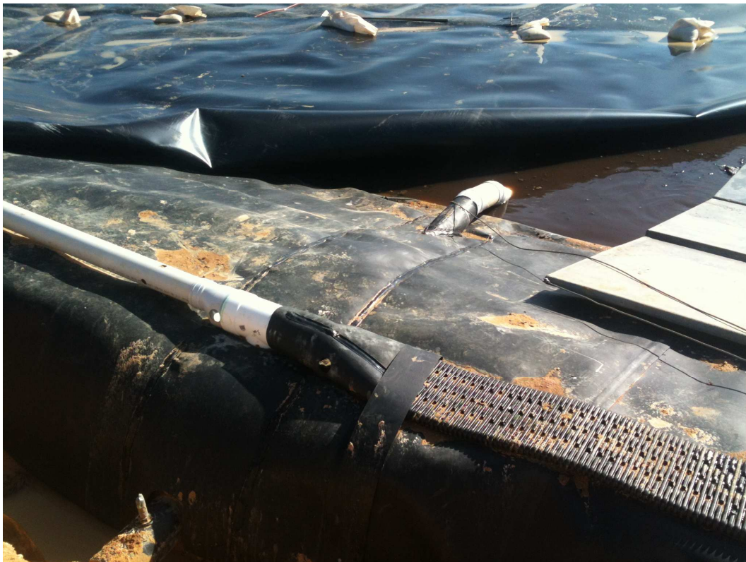
Figure 10: MegaFlo gas collection pipe
