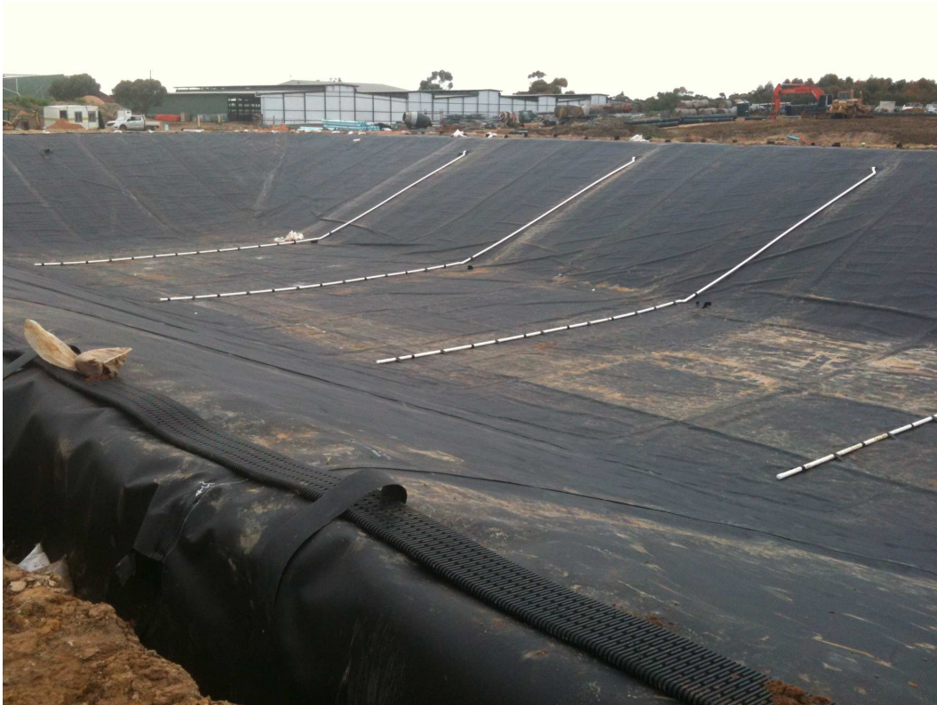
Figure 28: Lined eastern CAL showing sludge removal pipes and MegaFlo gas collection
