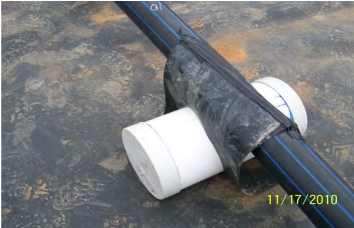
Figure 6: Weighting of Sludge Removal Pipes, AJ Bush Riverstone (Source: AJBush)
