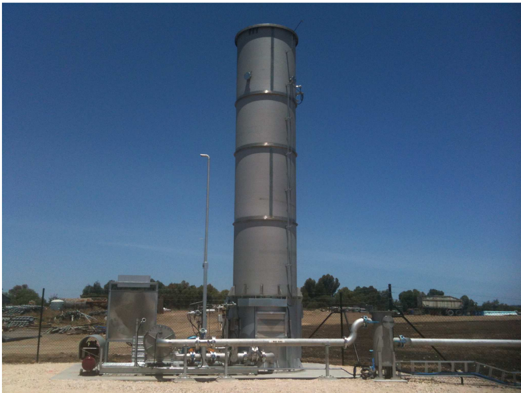
Figure 15: Installed gas train and high temperature flare
