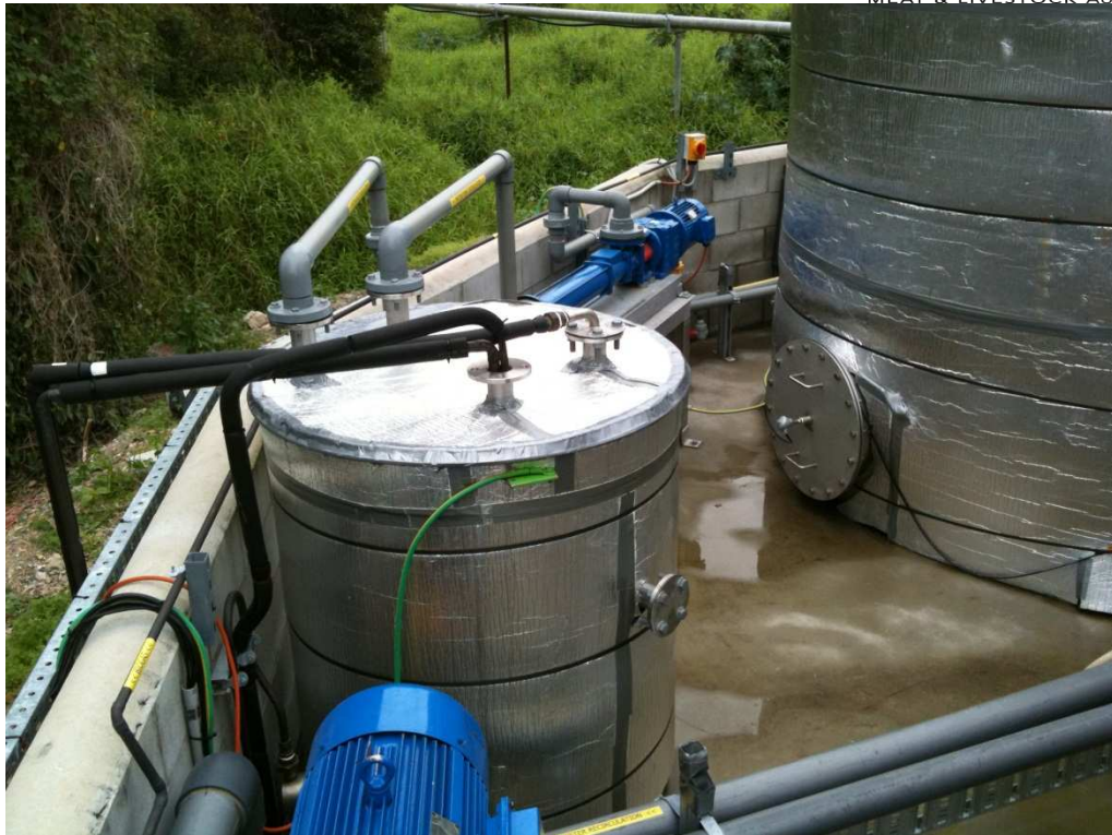
Figure 5: Shell and tube heat exchanger used to heat TPAD pre-treatment reactor
