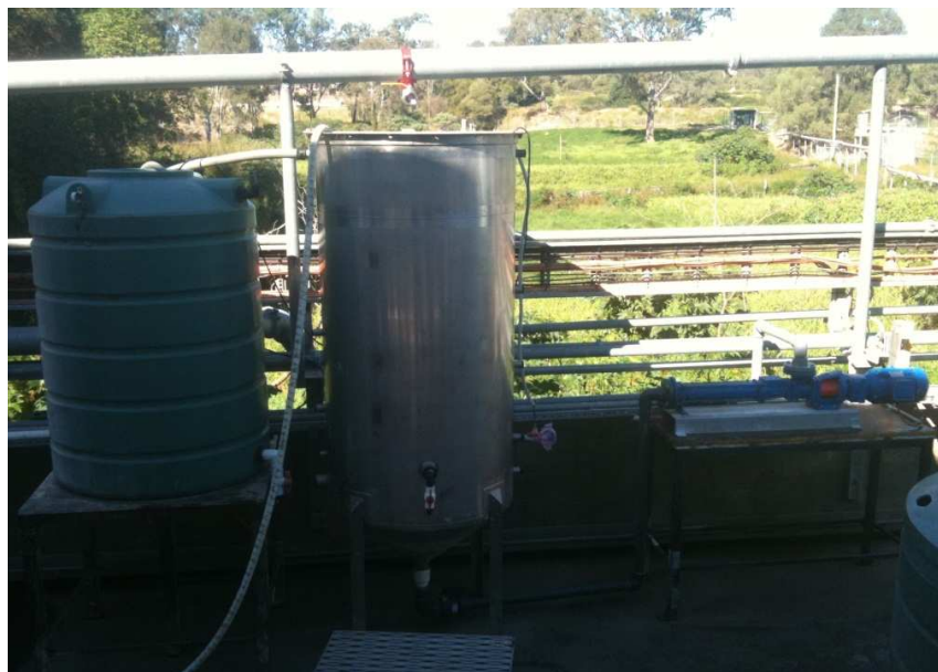
Figure 6: Wastewater feed collection system at TPAD demonstration plant host site in 2011.
