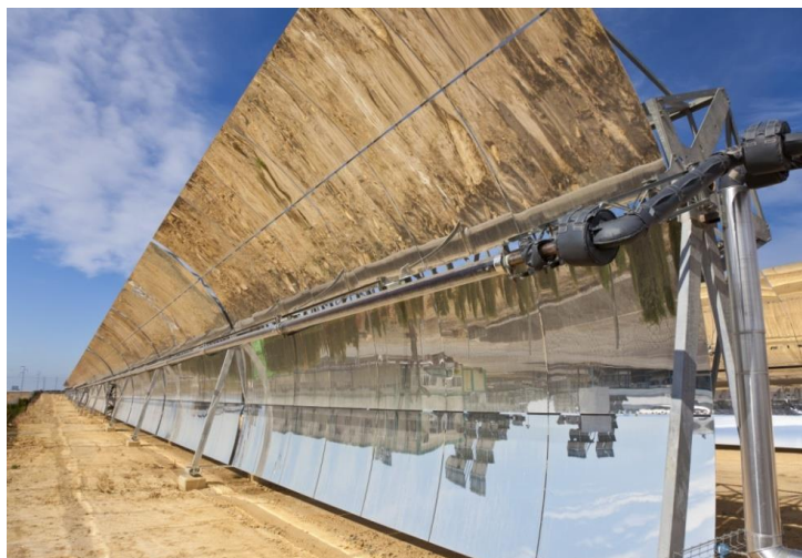
Figure 10: Mirrors at the Solar Energy Generating Systems plant in California, currently the largest solar thermal plant in the world at 350MW
