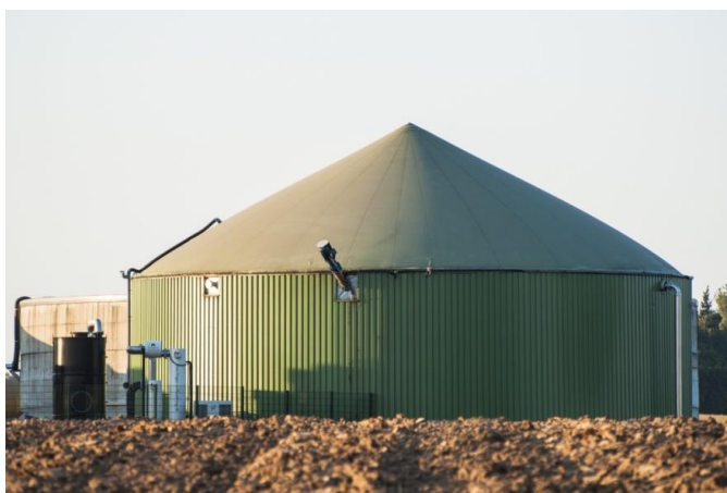
Figure 14: A covered anaerobic digester. This cover expands and can buffer gas delivery
