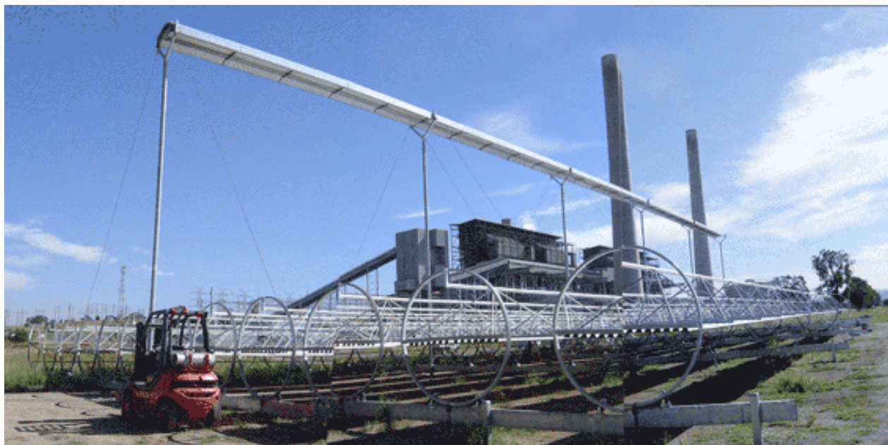
Figure 9: Liddell linear Fresnell array which supplies 10MW of steam to Liddell powerstation
