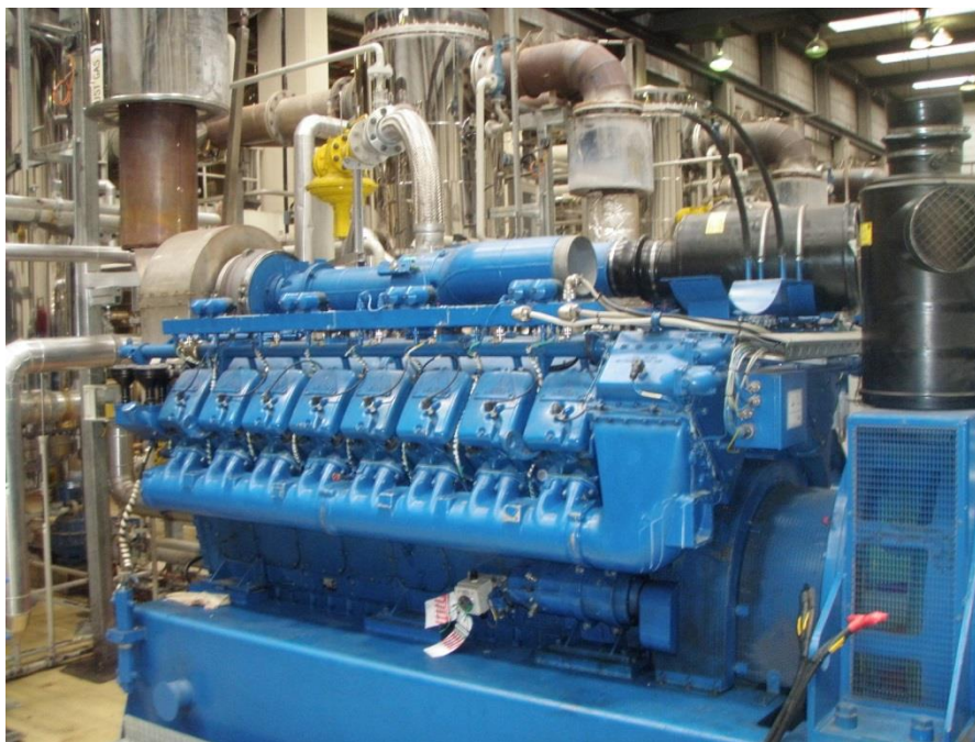
Figure 16: Biogas engine as part of a trigeneration system at a large sewage treatment plant
