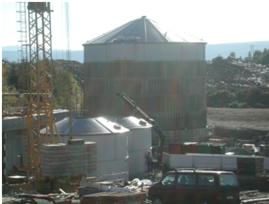
Figure 13 Storage for liquid carbon source and digester
