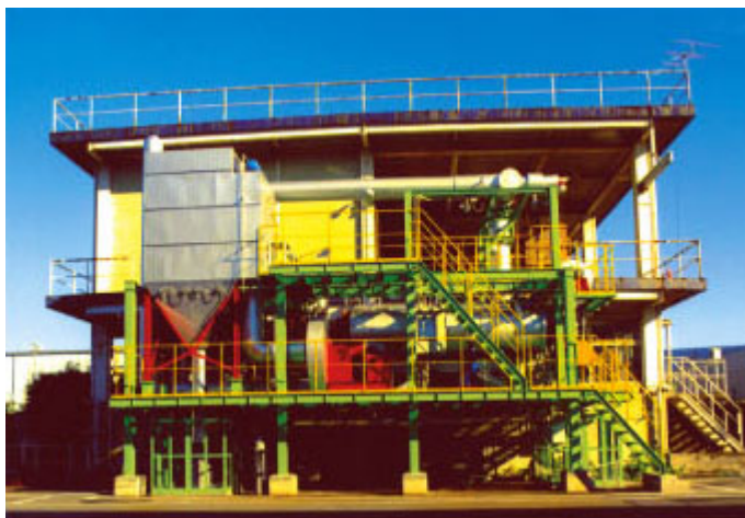
Figure 17 Pyrolysis system for municipal and industrial wastes at Honmoku Factory in Yokohama, Japan
