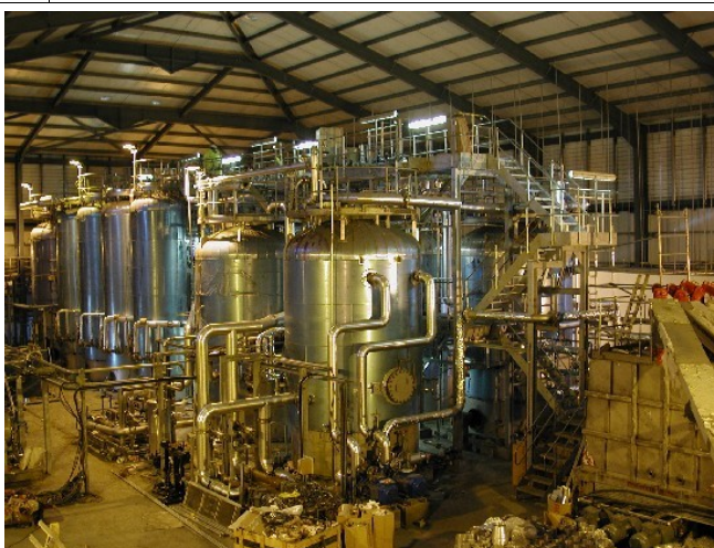
Figure 15 Cambi Thermal Hydrolysis Plant, Dublin
