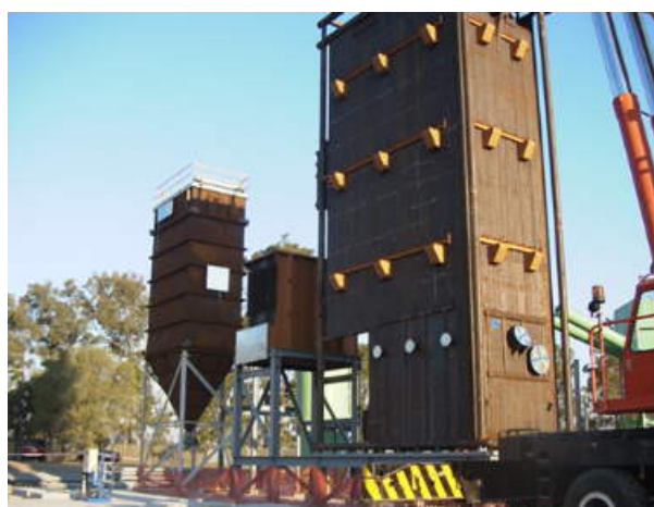
Figure 6 Fluidised bed combustion unit installed on green waste to energy site in Staplyton, Queensland
