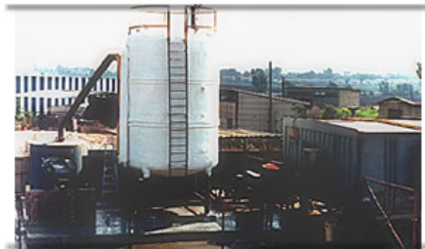
Figure 10 Anaerobic Methanogenic Thermophilic Digestion Unit
