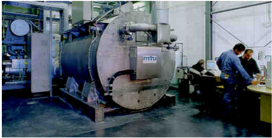
Figure C2 Molten carbonate fuel cell power plant
