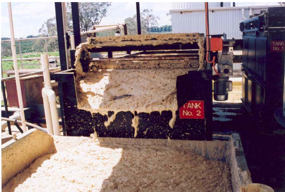
Figure 7: Sludge leaving separator 2
