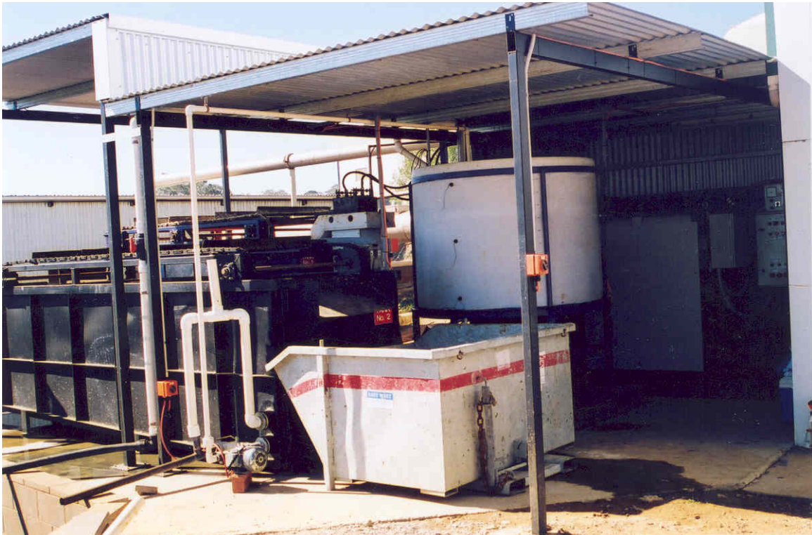
Figure 2: Electrocoagulation system at BMP, Young, NSW
