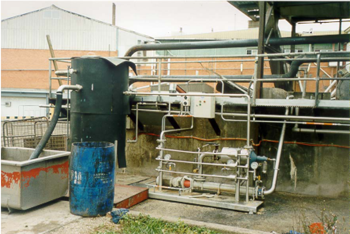
Figure 7 Meat Processing Plant No.2 – Hydrocyclone Installation
