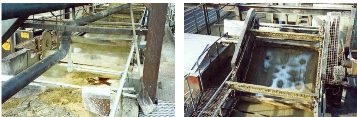
Figure 11 Save-all at Meat Processing Plant No.3
