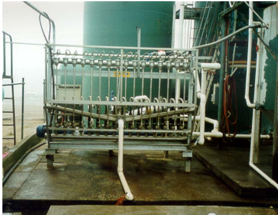
Figure 4 Meat Processing Plant No.1 – Hydrocyclone Installation
