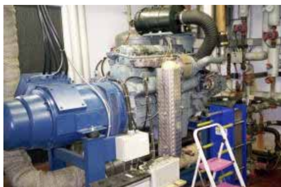
Gas engine, running on biogas
