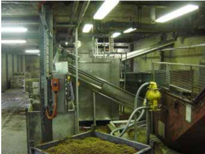
Dewatering screw system
