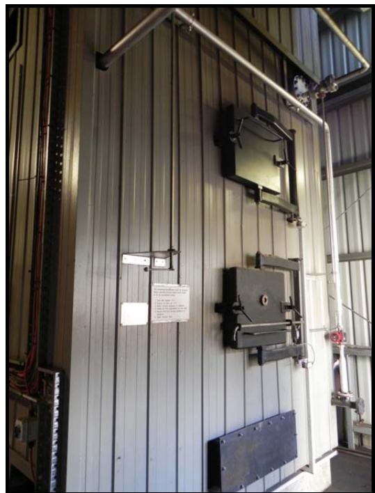
Boiler with inspection doors
