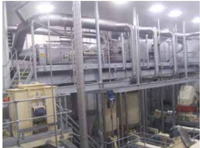
Ducting for odour control
