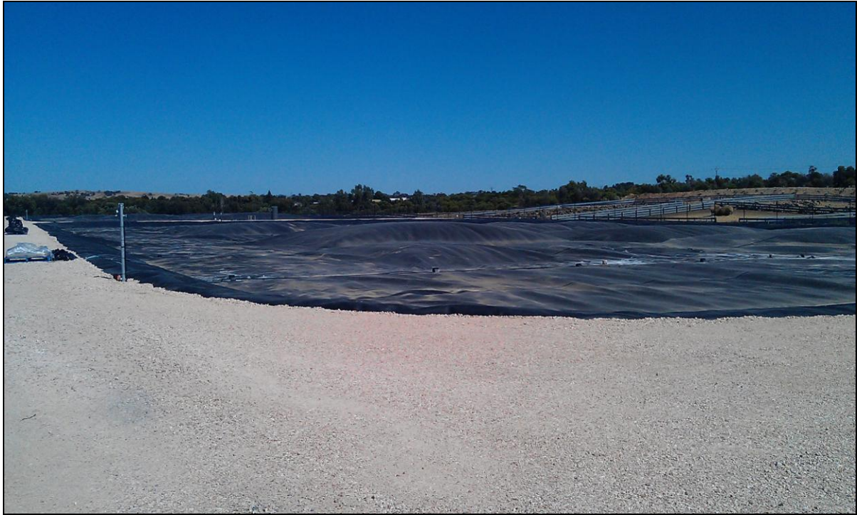
Photo 3.8– CAL system at Abattoir C
