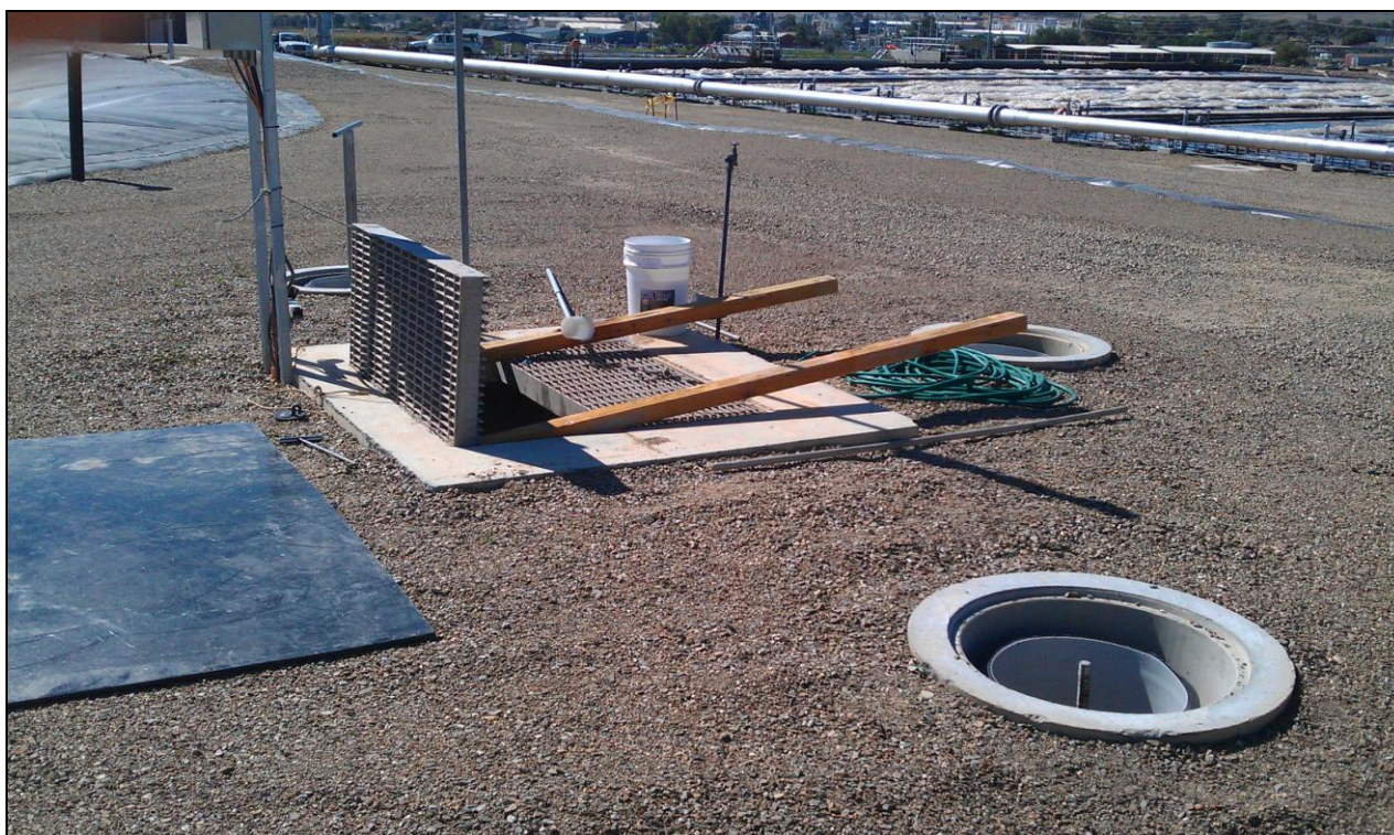
Photo 3.7 – Abattoir B: Outlet wastewater collection point
