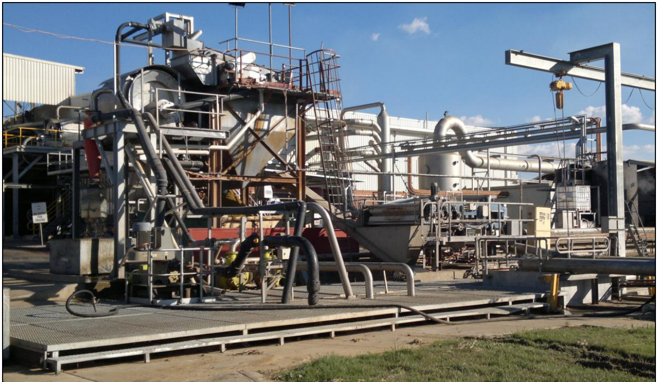
Photo 3.6 – Abattoir B: Inlet wastewater collection point
