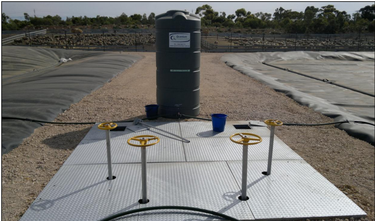
Photo 3.9 – Abattoir C: Inlet wastewater collection point
