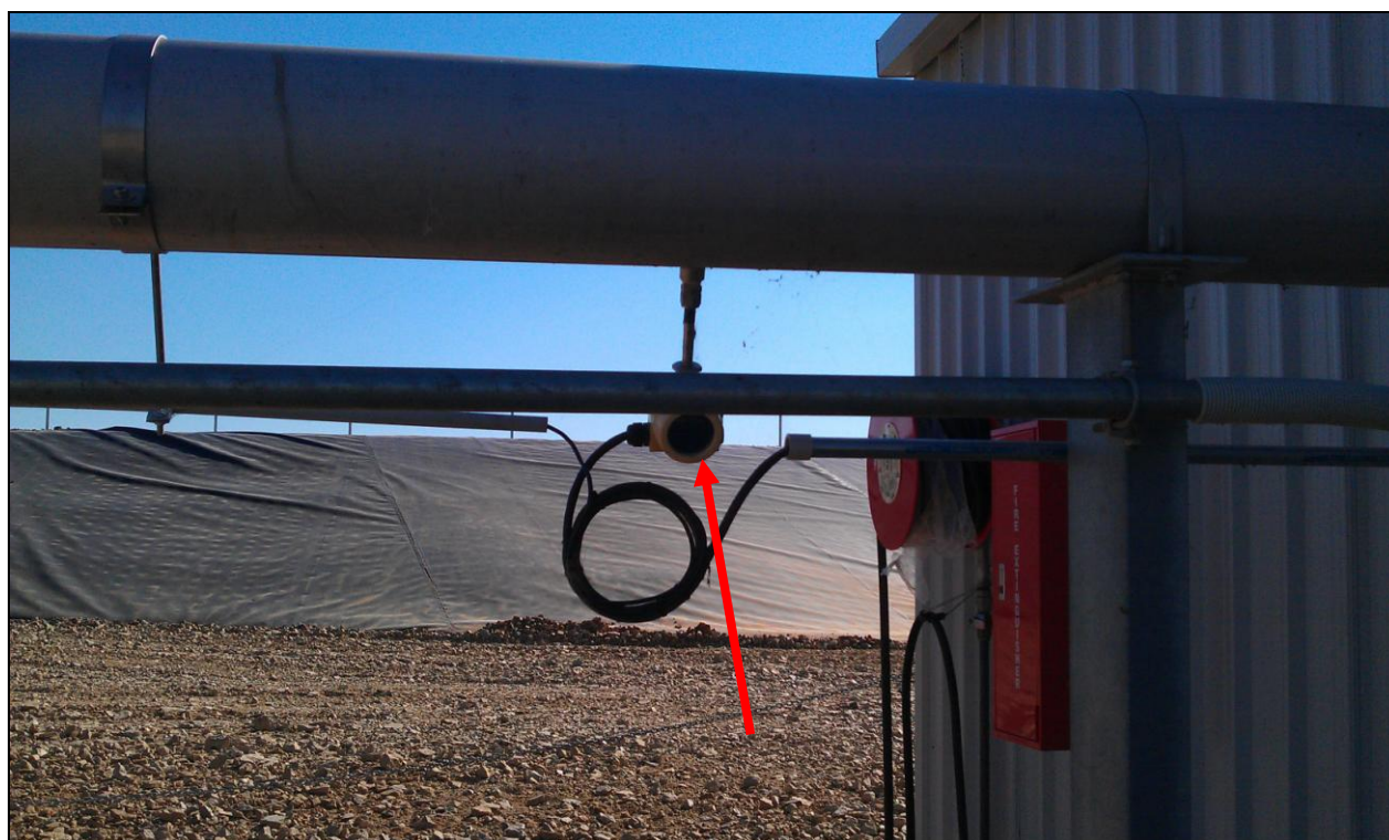
Photo 3.1 – Flow meter attached to the biogas flare system
