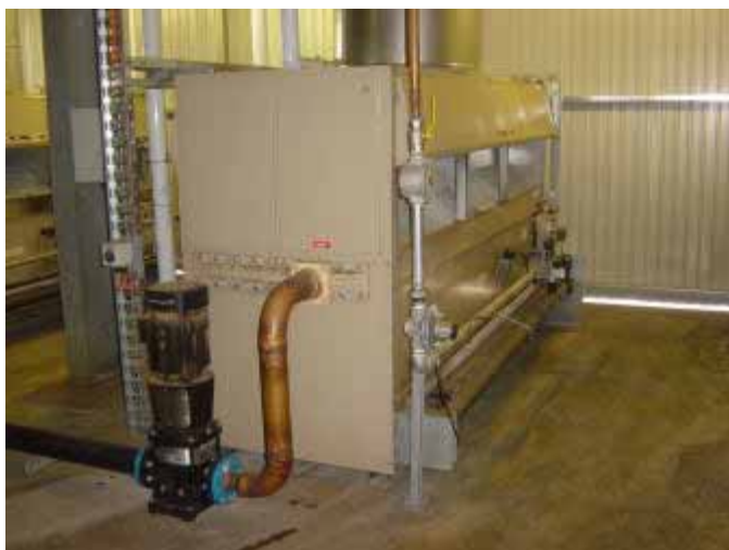
A hot water boiler is used where waste heat for hot water production is not available
