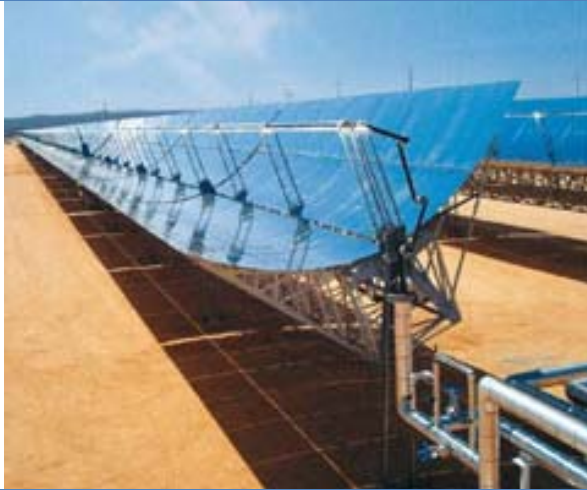
Parabolic trough collectors. The sun's rays are concentrated on a pipe containing the thermal fluid 27
