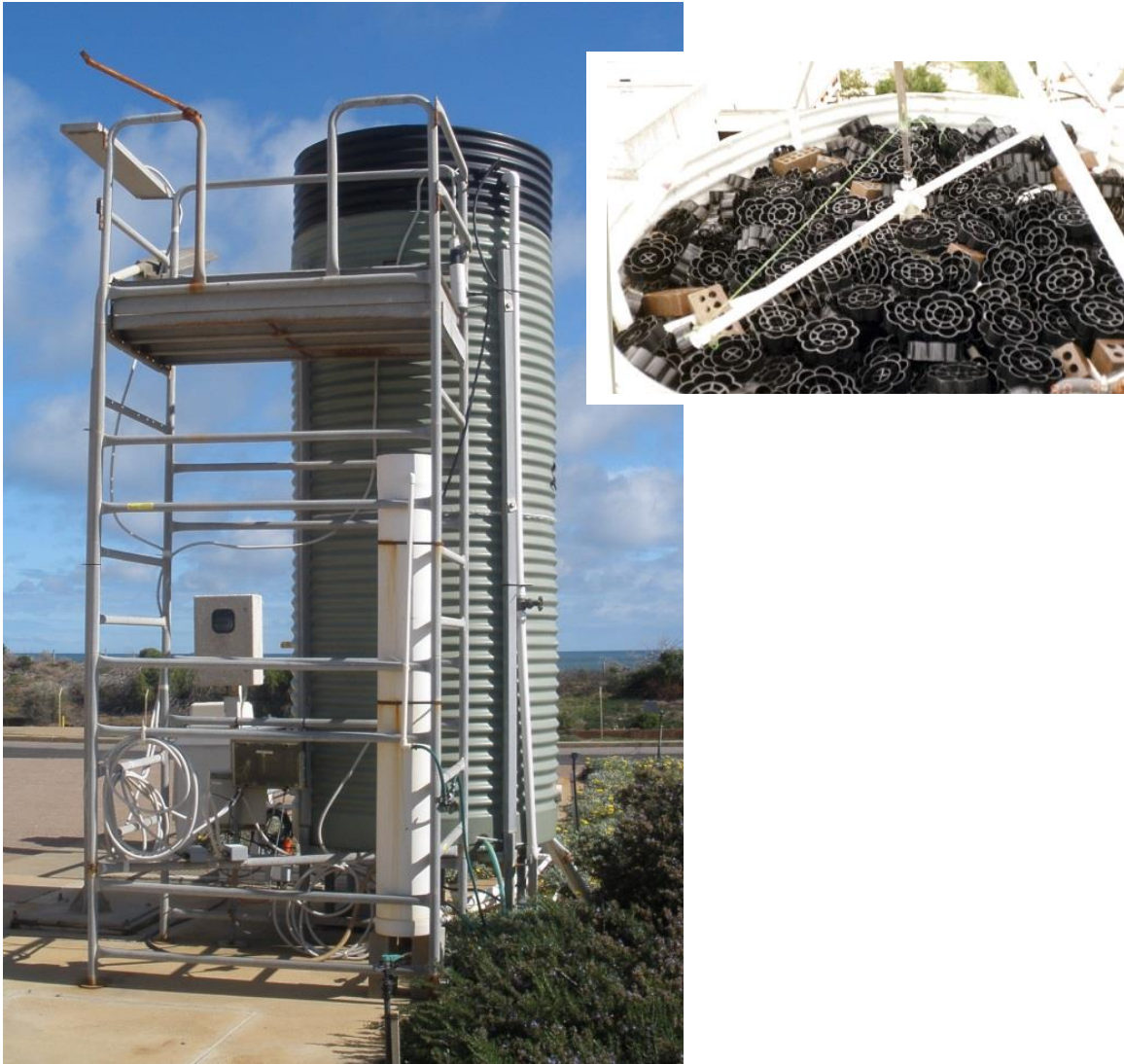
Figure 14: Example pilot plant trickling filters
