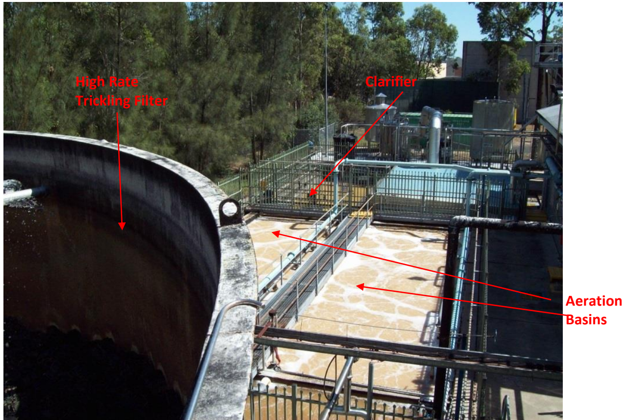
Figure 11: TF – Activated sludge process at soft drink manufacturer
