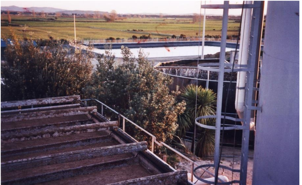
Figure 10: Chicken processing plant – TF downstream of DAF
