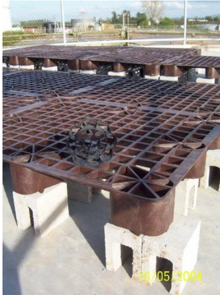
Figure 6: Underdrain support deck of trickling filter (space above floor of drainage collection slab should be about 0.4 – 0.5 m)
