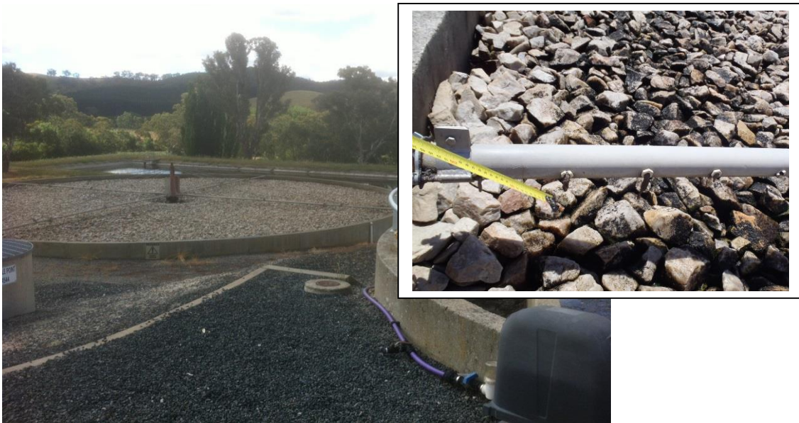
Figure 7: Blockage of distribution arm ports can lead to poor feed and drying out
